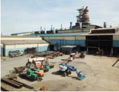
Construction zone for a new building to contain another oven at the Ohio foundry. April 2022 communications. Significant capital investments in our domestic manufacturing facilities have positively impacted our ability to service new and ongoing strong customer demand.
