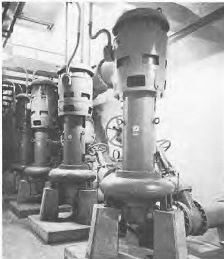
75 HP, 580 RPM, 6000 GPM Yeomans Raw Sewage Pumps in Municipal Pumping Station
