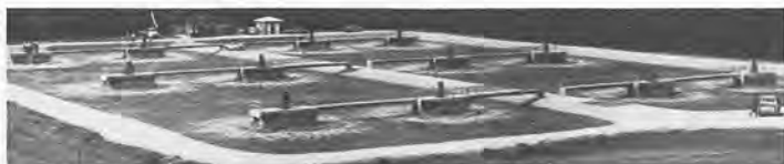
Twelve 75-H.P. Sigma Aerators treat difficult waste in a lagoon.
