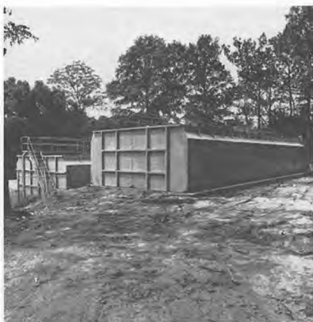
Subdivision duplex system—100,000 GPD capacity each plant.
