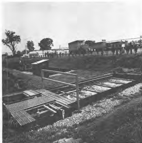
Truck Stop duplex system—20,000 GPD capacity each plant.
